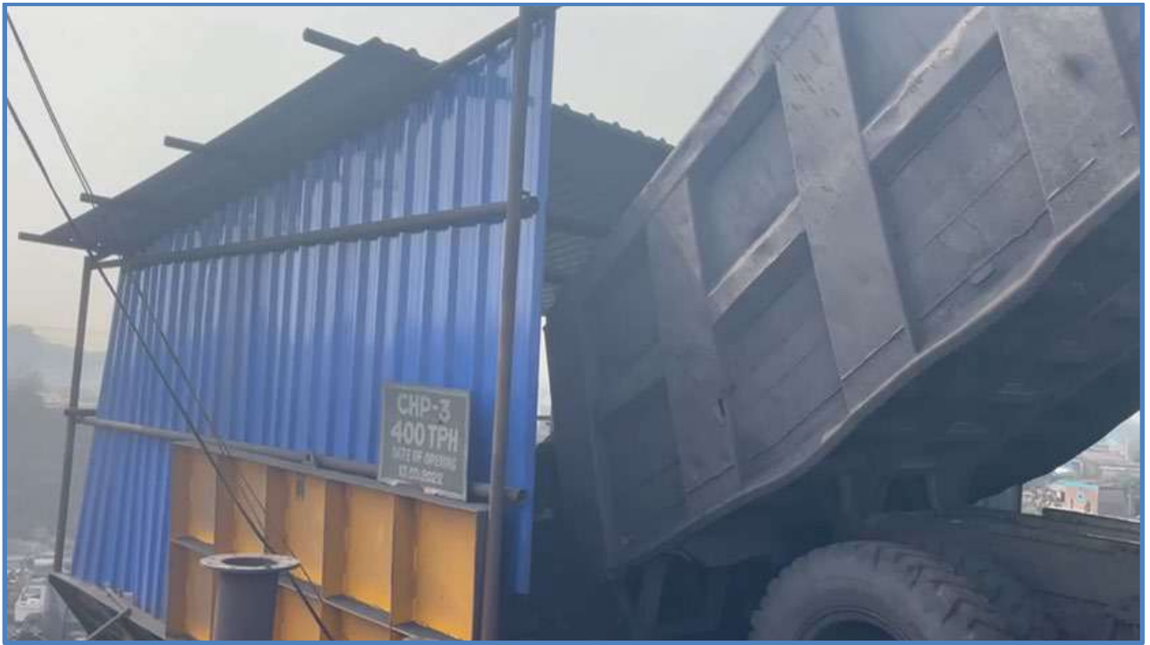
Picture 7 – Enclosed Coal Handling Plant
